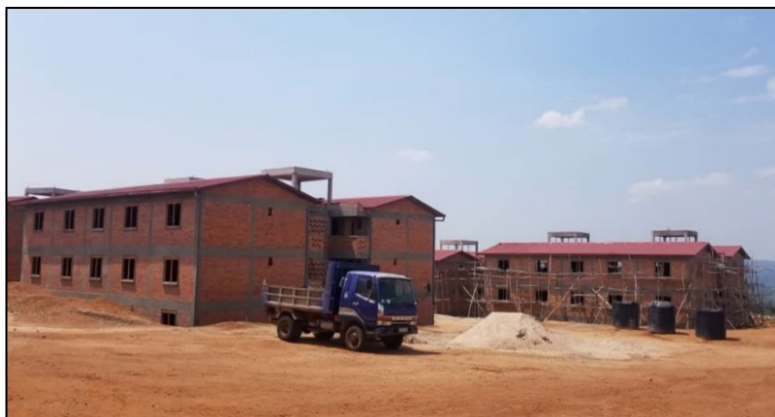
Figure 3.2. Construction of apartments for Kangondo residents at the Busanza resettlement site. Source: This picture was taken by Ernest Uwayezu in September 2019.
