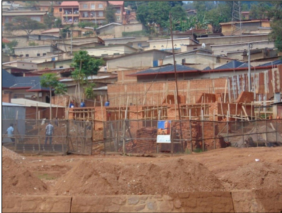
Figure 2.2: Construction of apartments for affected households at Mpazi research site, Source: Ernest Uwayezu, 2018
