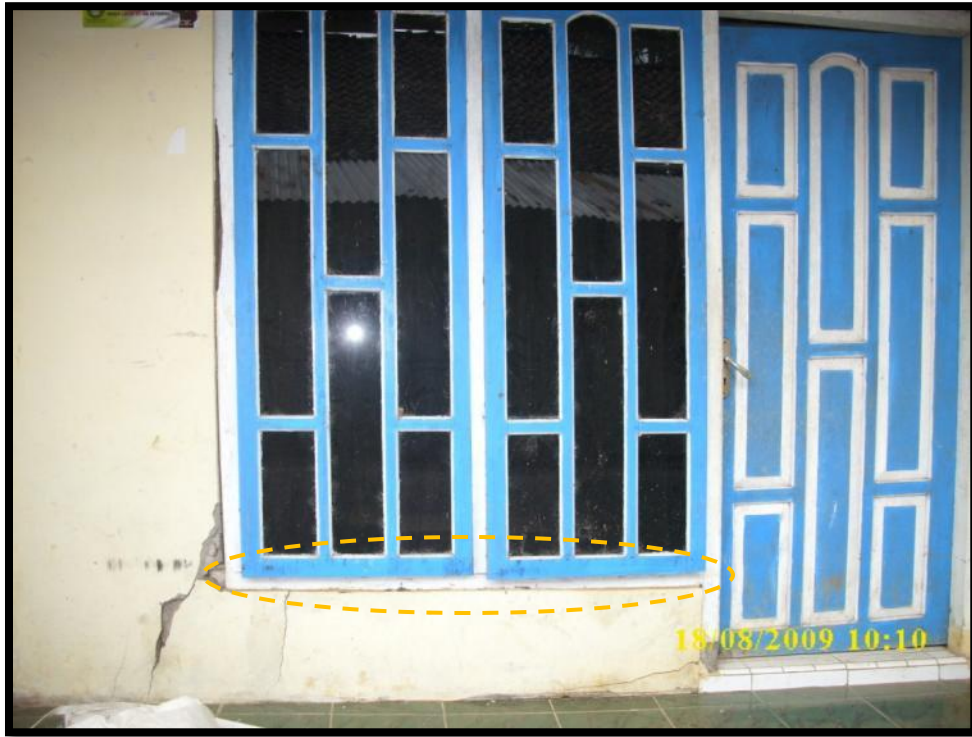
Creep. (Note the window blades do not fit to their frames anymore)
