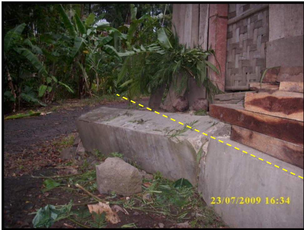
Creep. (Dotted line shows the house's original foundation position)
