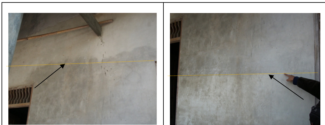
Figure 3.6. Flood marks in RT 3/RW 3 Kelurahan Joyotakan Left: Floodmarks of the 2008 flood; Right: Floodmarks of the 2007 flood. (source: fieldwork, 2009)
