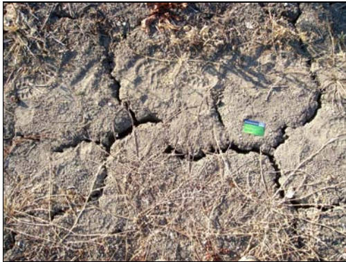
Photo B-2 - Cracks in topsoil due to high content in swelling clay
