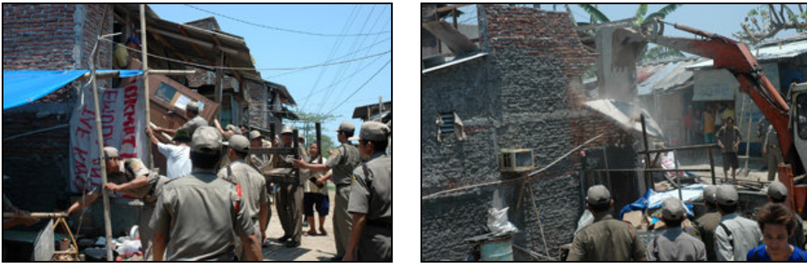
Figure 6-2: Clearance of informal settlement along the river bank of East Banjir Kanal by the local authority (Source: http://www.semarang.go.id , November 01, 2006)
