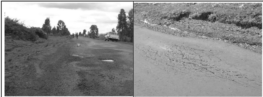
Figure 1-1: Problems of deformation and cracks on Addis Ababa - Jimma road sections (Netterberg 2001) due to the presence of expansive soils beneath the sub-grade.
