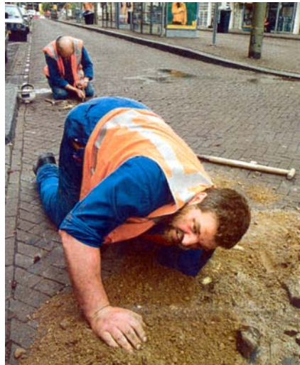
Figure 5.3: To avoid damage to cables, first digging by hand is necessary (Dutch Newspaper, July, 2000).
