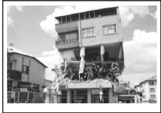
Figure 3.10. Total collapse of intermediate storey (Yoshimura, et al. , 2003)
