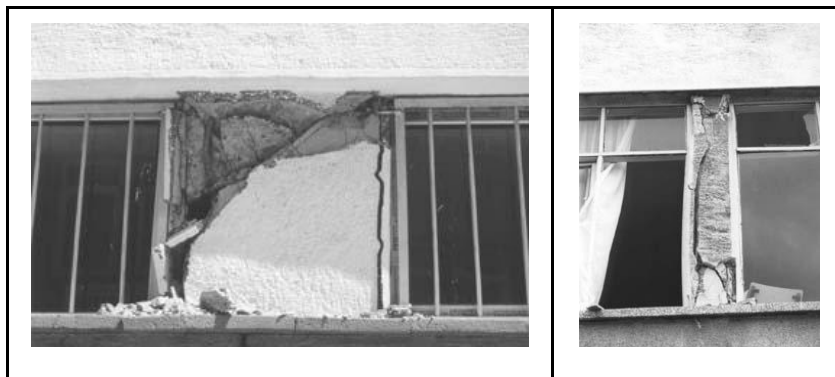
Figure 3.12. Shear failure in short captive columns ‘trapped’ between partial height infill, and flexural failure in non-ductile reinforced concrete plastic hinges (Bruneau, 2002)
