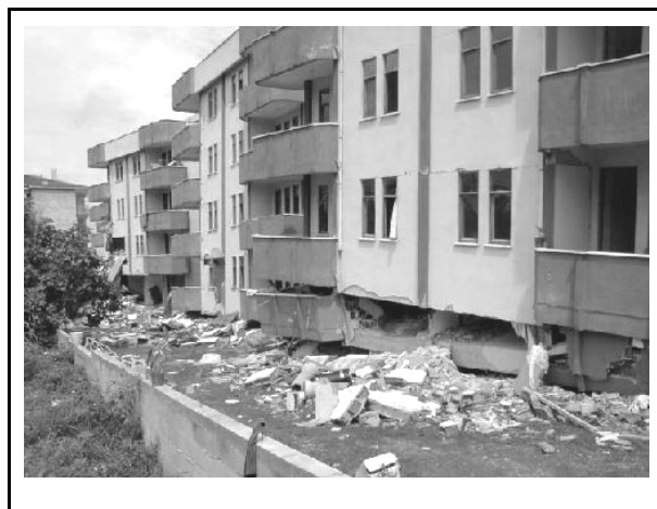
Figure 3.9. Damage due to soft first storey ( http://mceer.buffalo.edu visited on 14 November 2003)
